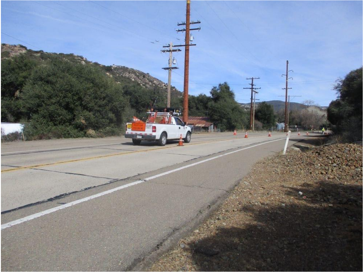
Photo 6: A pilot vehicle was used to lead one-way traffic through a coned off work zone on Old Highway 80 (TL 629A) in accordance with APM TRANS-02 and the TCP.
