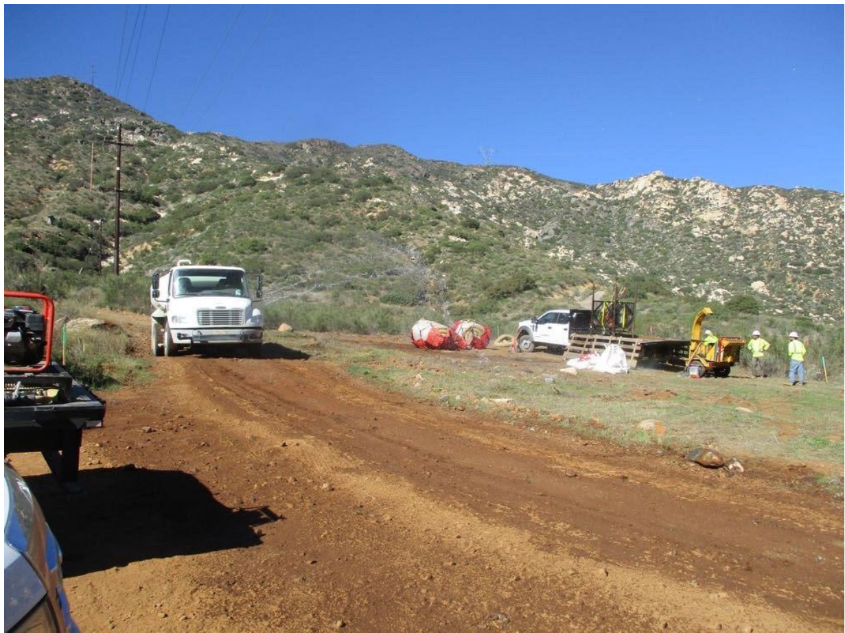
Photo 1: A water truck operator was observed applying water to the work area at SS03 (TL 6923) to prepare for helicopter external load operations (transporting equipment) in accordance with APM AIR-02.
