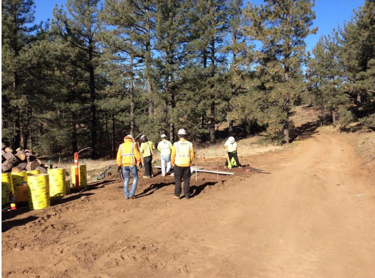
Photo 4: Archaeological and Cultural Monitors were present to monitor bollard excavations at a box location along Alignment C (C 440) in accordance with the HPMP, APM CUL-04, and MM CUL-1.
