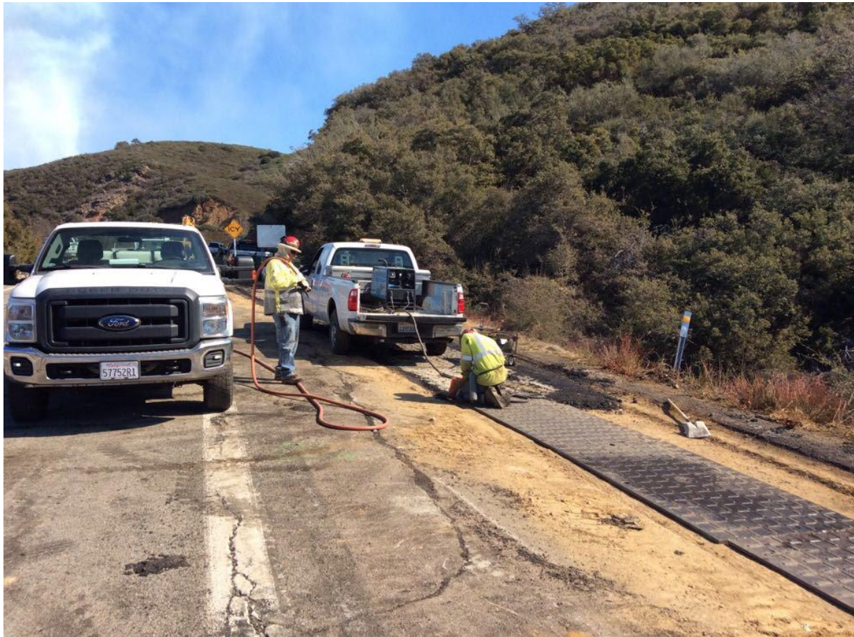
Photo 5: In accordance with the CFPPP, a Dedicated Fire Patrol was present during hot work near station 183+50 (C 440) and remained on site for one hour afterwards. The Fire Patrol was equipped with a full set of fire tools (5-gallon backpack pump, round point shovel, Pulaski, and 2A10BC fire extinguisher) and was also observed wetting down the surrounding area prior to hot work.
